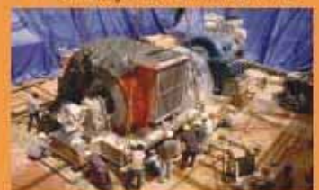
▼ TPI Ethylene - Steam Turbine
