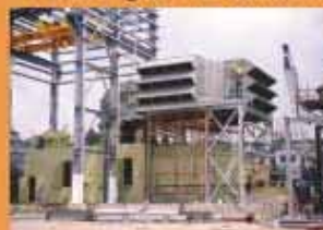
▼ BKK Cogent - Gas Turbine 6FA
