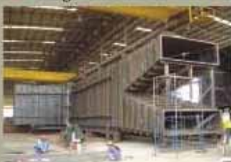
▼ Rabigh - Boiler Duct
