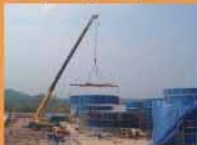
▼ Sepon Copper-Duplex Tanks
