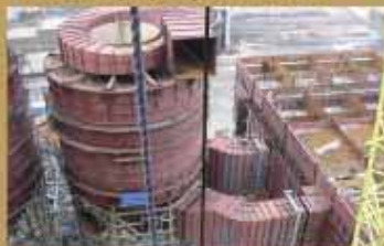
▼ AEP - Spray Dryer Absorber
