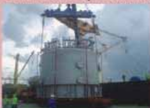
▼ Shadeed DRI - Top Gas Scrubber
