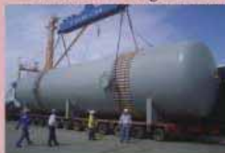
▼ Shadeed DRI - Purge Gas Tank
